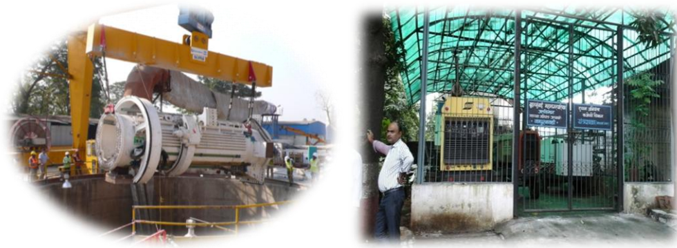
Site Visit: Bhandup Water Tunnel Project at Kapurbawdi, Mumbai For VDCE Student
