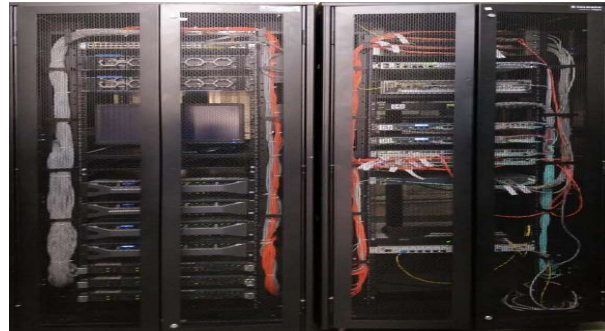
Server and Network racks in the CCF-1 Datacenter of VJTI
